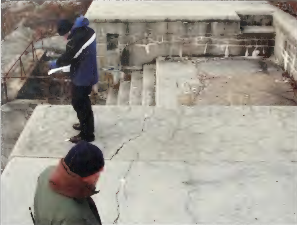
Figure 5.27. View looking down at gun platform #5, Battery Urmston. The tops of the magazines and bomb proofs show less evidence of spalling concrete, yet substantial cracks are present (Olmsted Center, January 2009).
